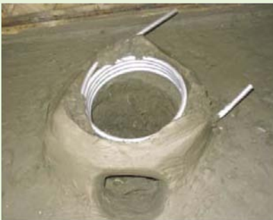
Photo 8: Construction of a flow-through system in a traditional Bangladeshi clay oven. (Source: Richard Johnston, UNICEF in Fakhrul Islam et al., 2006)
