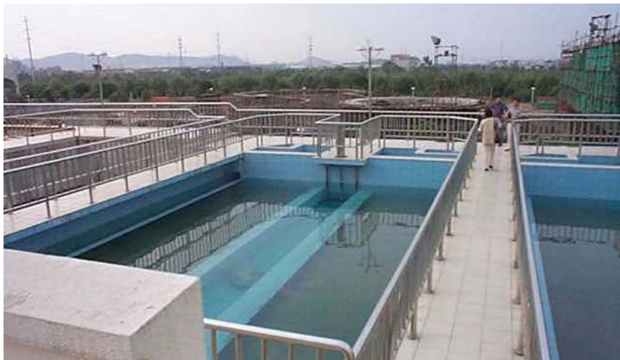
Photo 3: Water treatment plant. (Source: Courtesy of WEDC, © Sam Godfrey)
