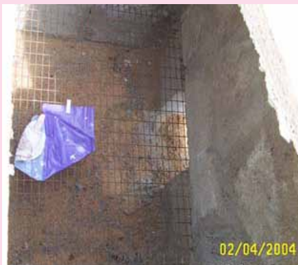
Fire grill inside incinerator
