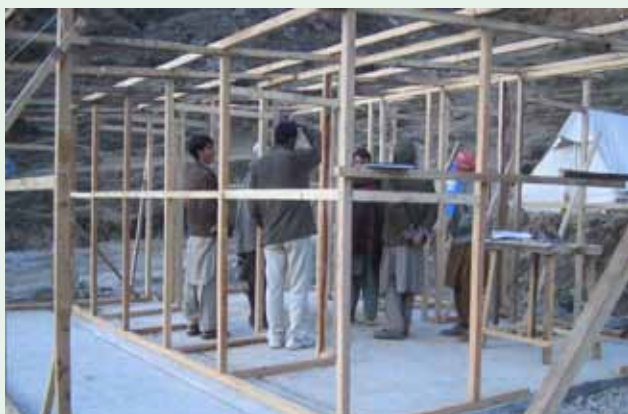
Warm bathing unit under construction – laundry area seen to the left of the picture
