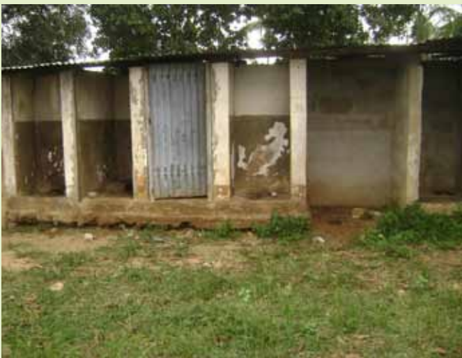
Over 50% of girls' latrines had no doors (Photos: Geodata, Tanzania)
