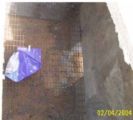
Fire grill inside incinerator
