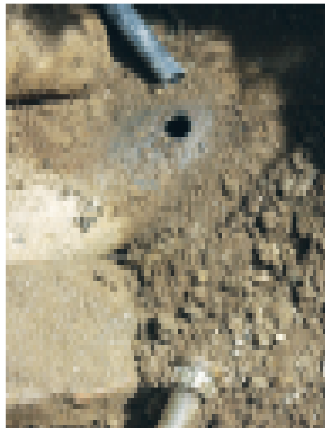
Illegal connection in Nepal
