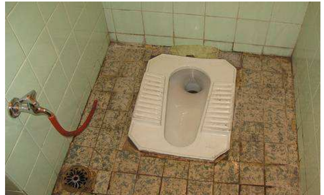
Fig. 5: Typical toilet in Syria: Squatting type with flushing. Hose on the left is for anal washing with water. Source: E. v. Münch, Jan. 2009.
