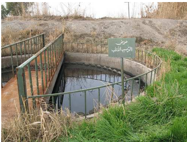
Fig. 7: Circular primary settling tank at Haran Al-Awamied treatment plant. Source: E. v. Münch, Jan. 2009.
