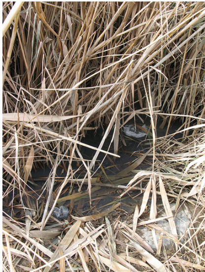
Fig. 9: Overloaded, water-logged reed bed towards outlet section of reed bed (source: E. v. Münch, Jan. 2009)
