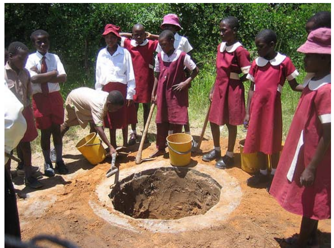
Figure 1: Pupils at a school in Epworth, Harare in Zimbabwe learn to build their own toilets: digging the shallow pit of an Arborloo inside a concrete ring beam (source: Aquamor, Zimbabwe, 2009). More photos of this school available here: www.flickr.com/photos/gzecosan/sets/72157626300000229/
