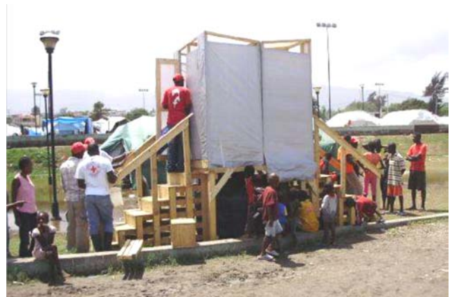
Figure 1: Raised toilets in Haiti provided by IFRC for 275,000 people per day with materials produced in Dominican Republic and constructed in Haiti (source: IFRC, 2010).
