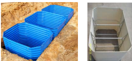
Figure 7: Emergency pit lining kits to avoid collapse. A man hole provides access for desludging. Left: modular corrugated plastic. Right: new design with internal props (instead of relying on locally available wooden props included in former design (source: J. Rhode, Evenproducts, 2011).
