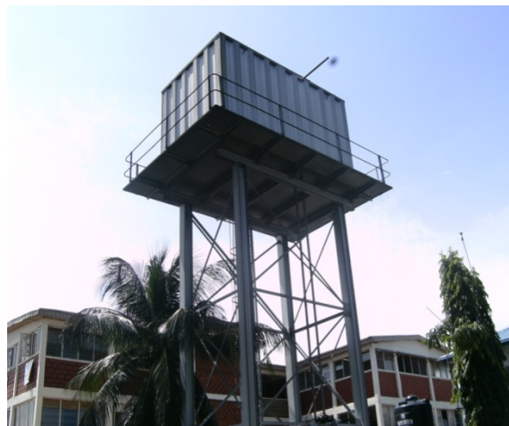
Plate 2: An overhead water tank servicing the a formal water vendor
