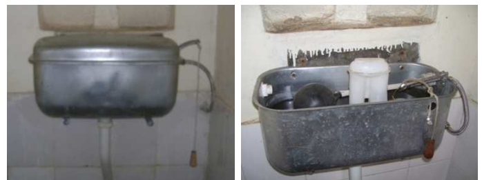
Fig. 13: Cistern after installation (left) and after vandalism/misuse and theft (right) a few weeks later. Repairs were undertaken by WSP, but the toilet operator now shifted to a pour flush system.
