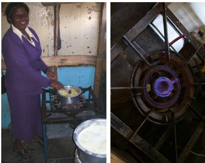
Fig. 12: Biogas is used to cook snacks and tea at the adjacent cafe.
