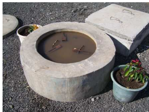
Fig. 8: Area of the top manhole (above biogas fixed dome) of the biogas plant. Clay is used for sealing the lid, and water to keep it wet and thus detect leakages that would show up as bubbles.
