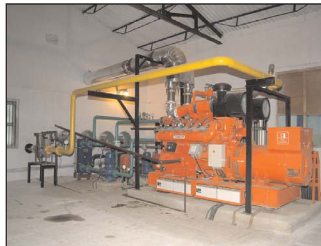
Biogas Engine Generator & its Auxiliaries
