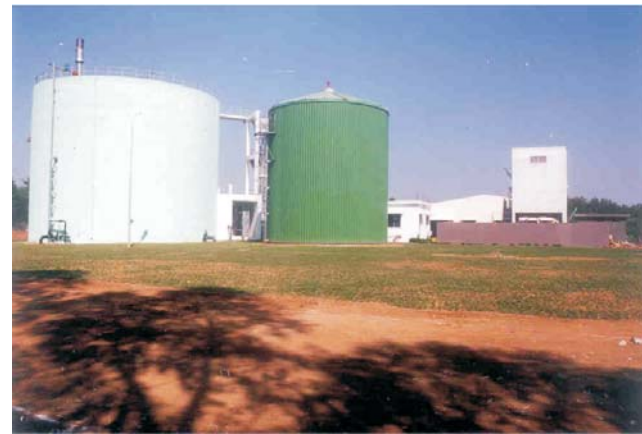
Biogas Digester and the Gas Holder
