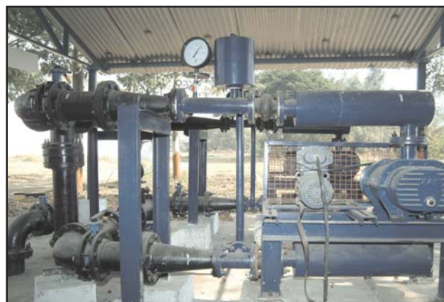
Biogas collecting Blowers and its piping
