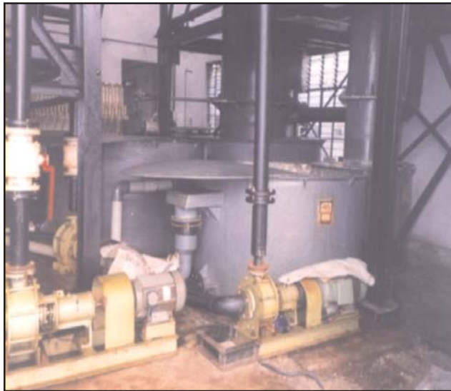
Scrubber and Pumps
