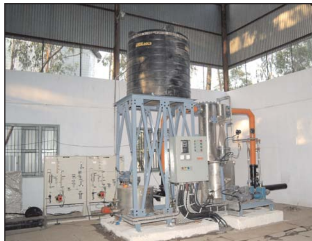
H 2 S Scrubbing System
