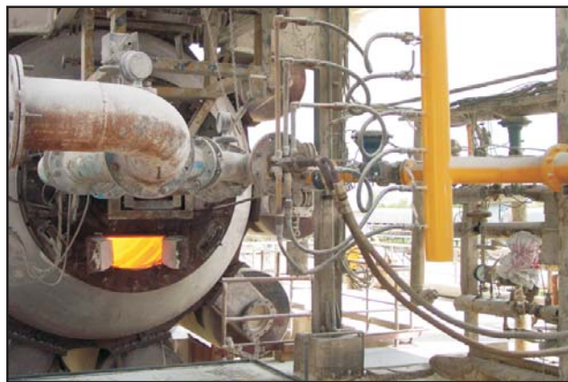
Gas firing in Lime Kiln
