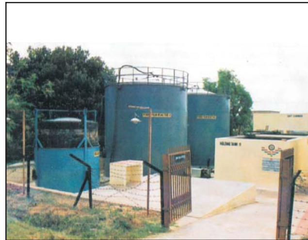
Fixed Film Reactors and Biogas Holder
