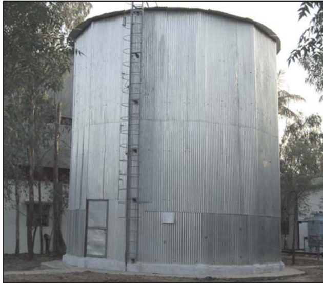
Biogas holder with MS protection Silo
