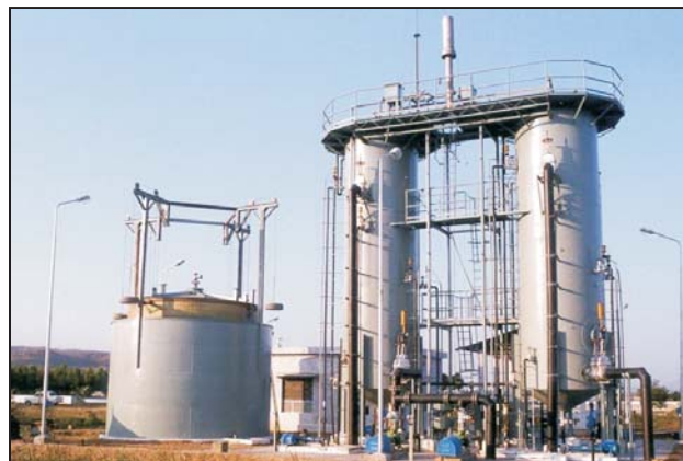
Fig. -1 Two Digesters and the Gas Holder
