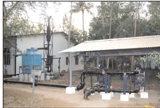
Biogas Blowers for Engine, Cooling Tower
