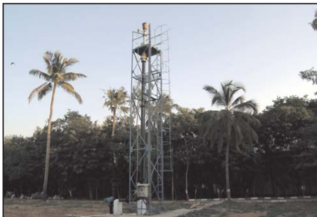
Biogas Flaring System
