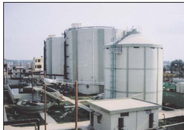
Two BIMA Digesters and the Gas Holder
