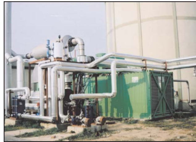
Gas Engine with associated piping network
