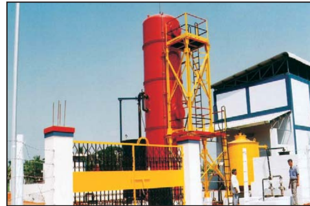
Biological Scrubber for Removal of H_2S
