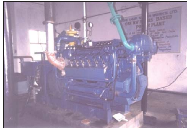
One of the 300 kVA Gas Engine from M/s. Greaves
