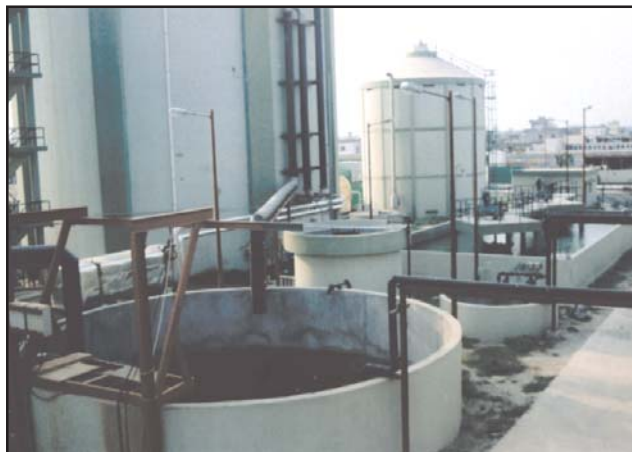
Effluent Treatment Plant
