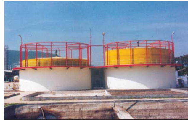
Anaerobic Digesters (HUSMAR)
